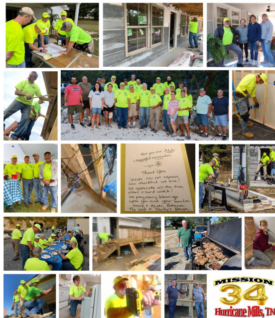
ST. LOUIS SLUGGERS 28 of our St. Louis Sluggers just returned from their fourth trip to Humphries County, TN. Work was on flood recovery operations and building a homeless village. They were hosted and assisted by the local St. Vincent de Paul Conference. Heavy lifting was by trustees from the Sheriffs Workforce. Mission 35 is scheduled for mid-April 2024.
